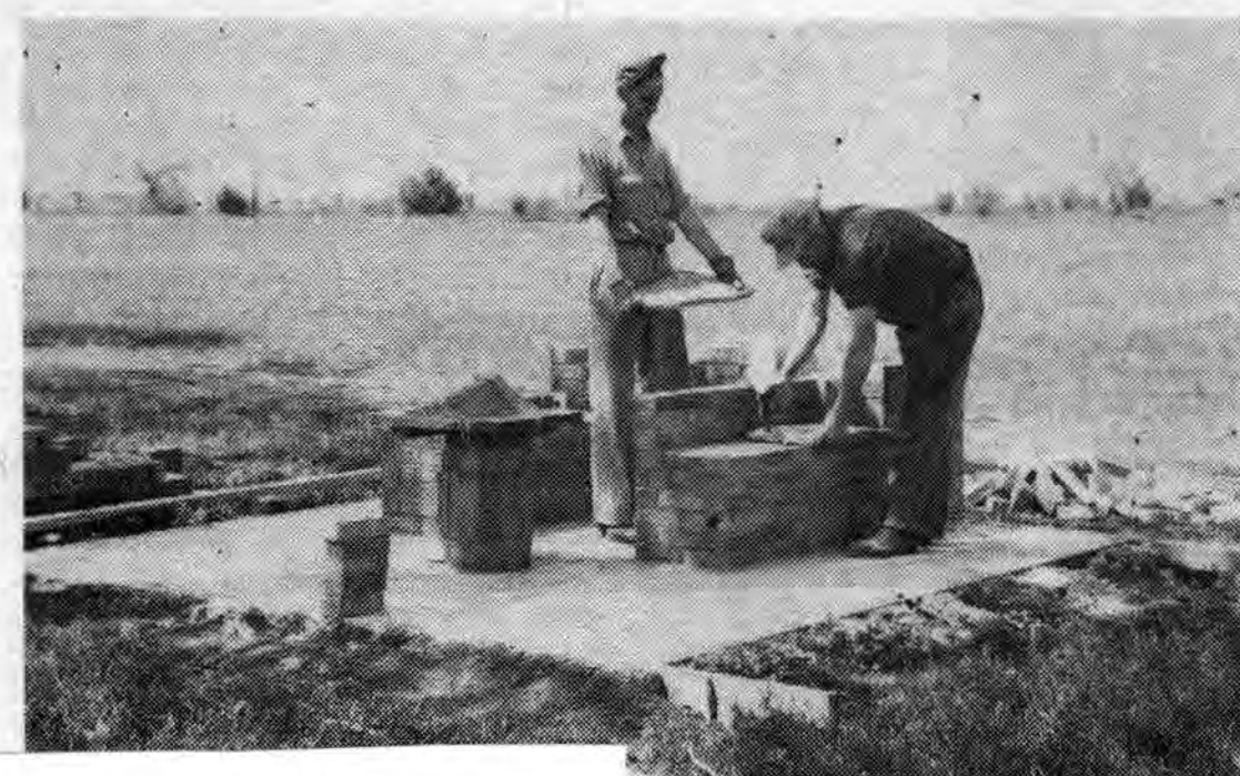
Ted Martin and Willard Rogers are shown constructing the dutch ovens which are being built in the park. The ovens are constructed over a concrete slab to assure and prevent the possibility of fire from the ovens. Mr. Martin is laying a stone slab on top of the oven and the ovens for the top of the oven are being constructed. The hamburger and wiener will "taste" good.
