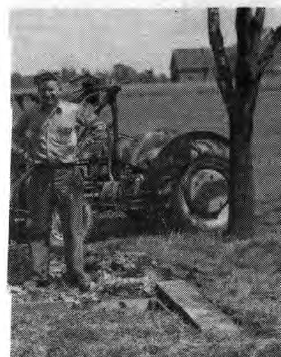
The foundation on which will be erected the "Chic" Sales. Herman Westover, Charley Brinkman and another man are shown laying the foundation for the restrooms, located near the dutch ovens. It will be the responsibility of all employees to keep the rest rooms in a clean and sanitary condition.
